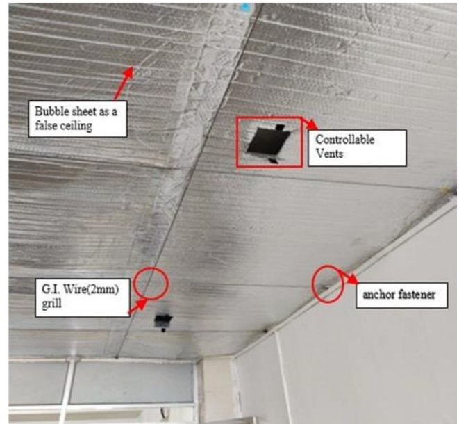
Fig 1 Inside view of installation in room No. B-341.
