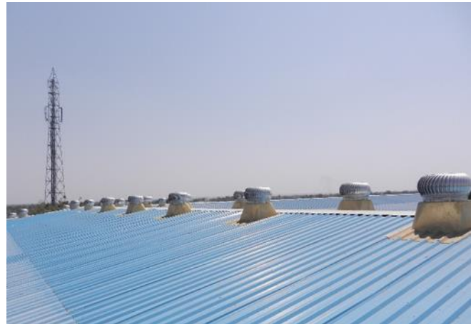
Fig. 2 Outside view of turbo ventilators on sheet metal roof top of the building.
