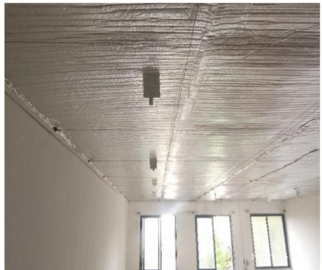
Fig.3 Inside view of installation in room No. B-341.
